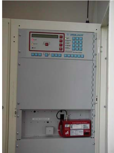
Figure 8: Typical Fire Indicator Panel Installation
