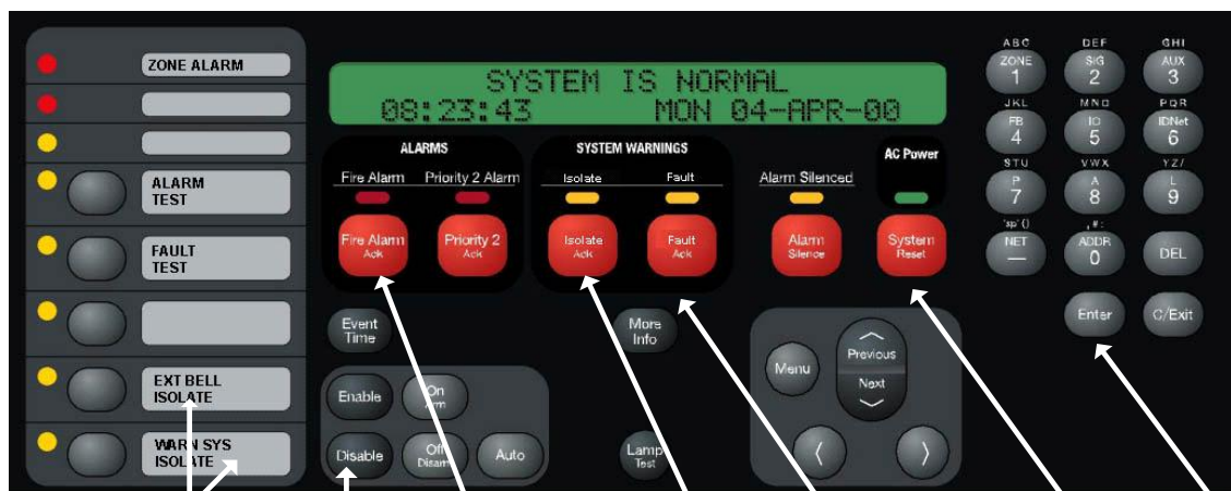
OUTPUT ISOLATES DISABLE FIRE ALARM ACK ISOLATE ACK FAULT ACK SYSTEM RESET ENTER
